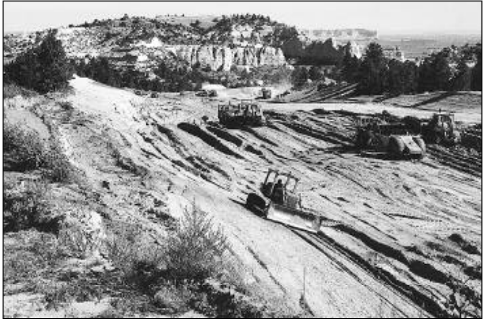
During construction, heavy equipment prepared the landscape for the new roadbed of the Gering South project.
